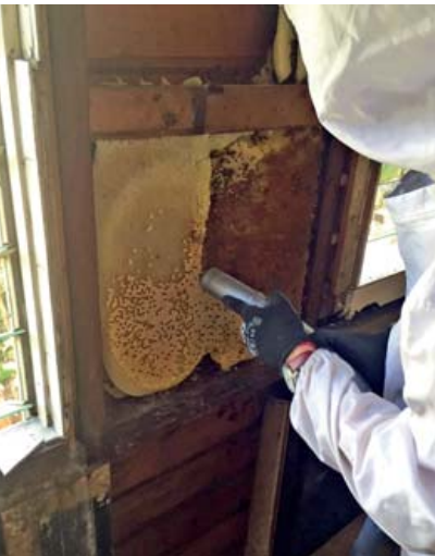
Swarm of bees being removed from a wall cavity during a Hutchies' house demolition in Highgate Hill.
