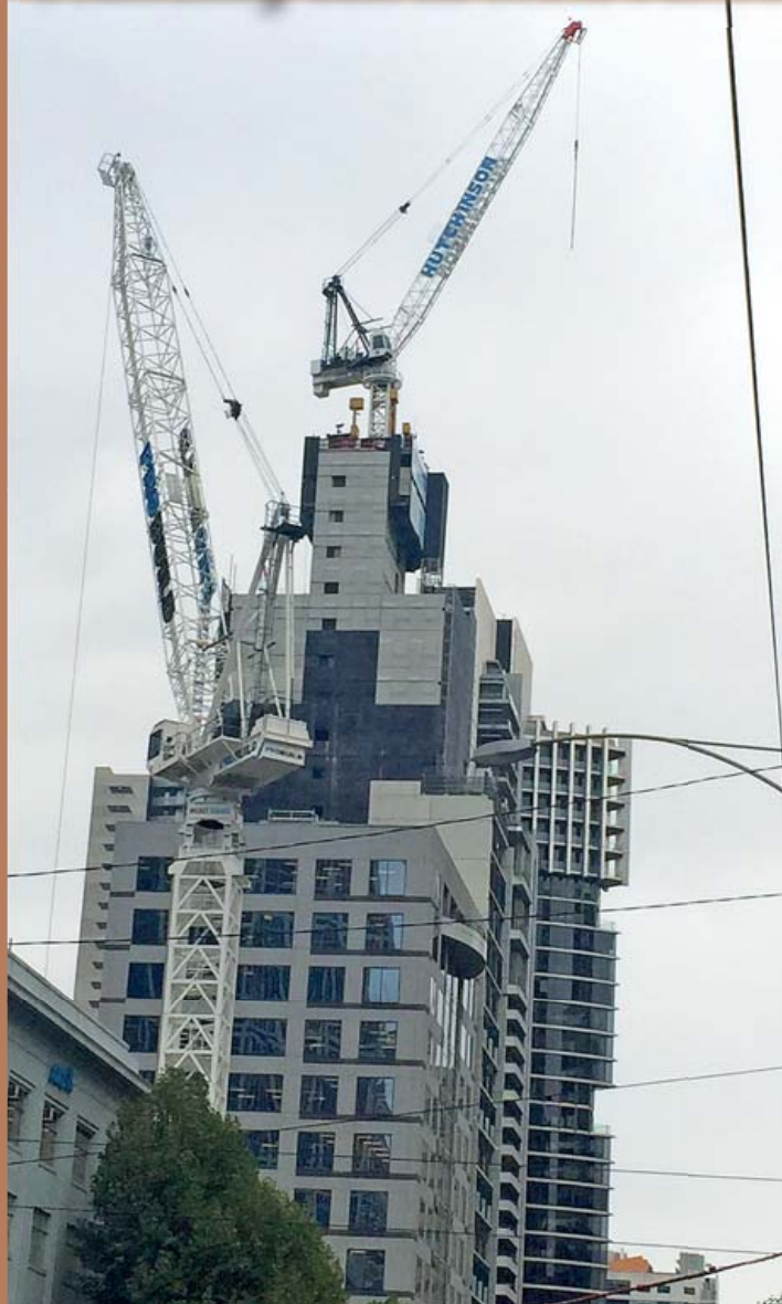
HUTCHIES' name is standing tall in the Melbourne CBD as the $34 million Carlson Apartments building in La Trobe Street tops off at 35 storeys. The 149-apartment residential tower is due for completion in December.
