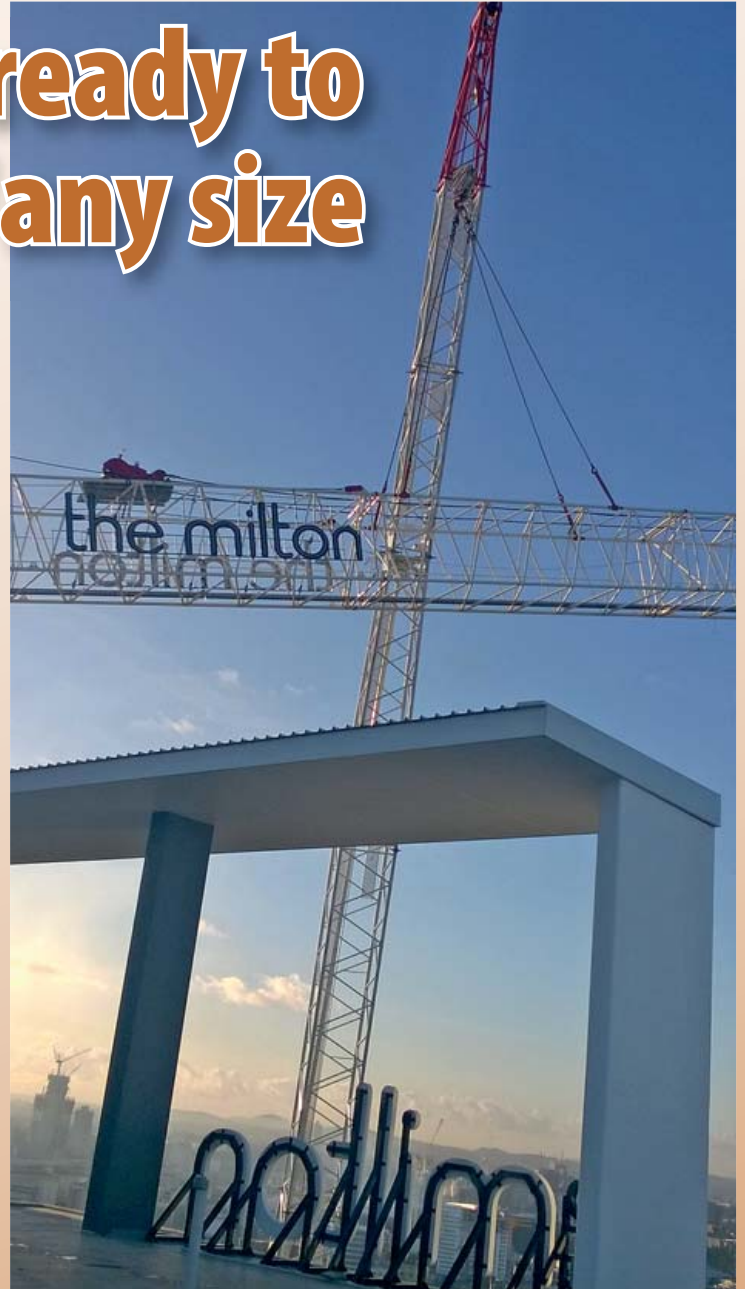
Hutchies' Milton crane which has been a feature of the Brisbane inner suburban skyline has gone, with completion of this major project. Image shows the Milton crane being taken down.
